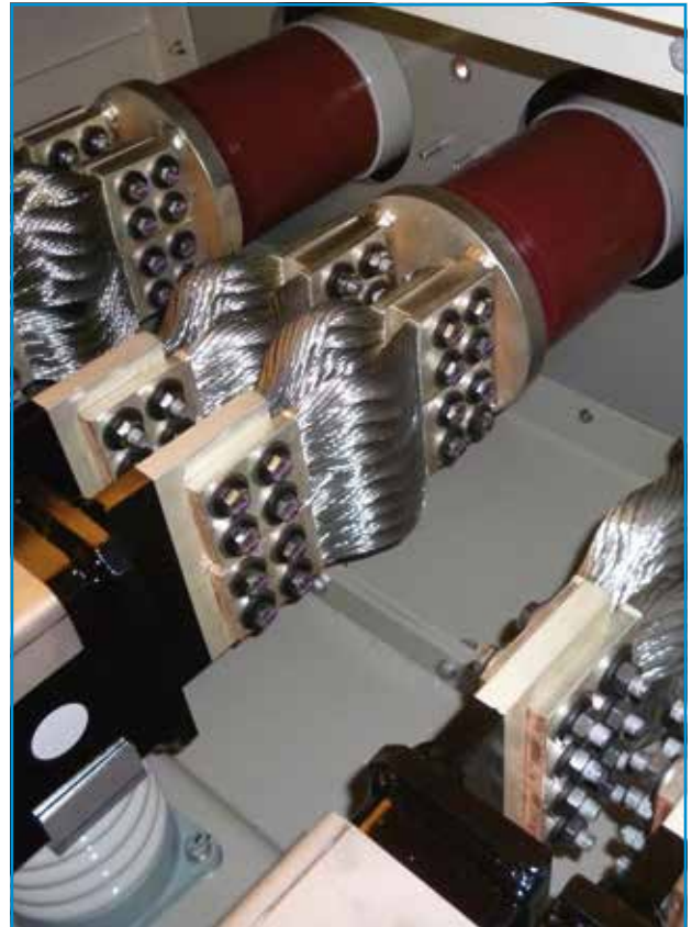
5000A generator connection
