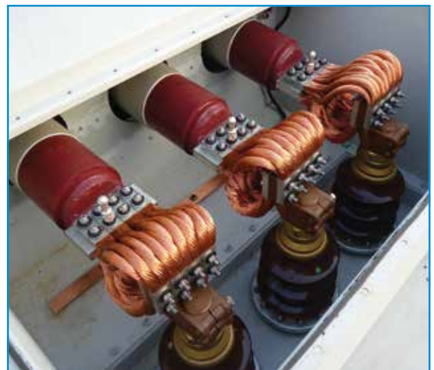
Copper braids to transformer
