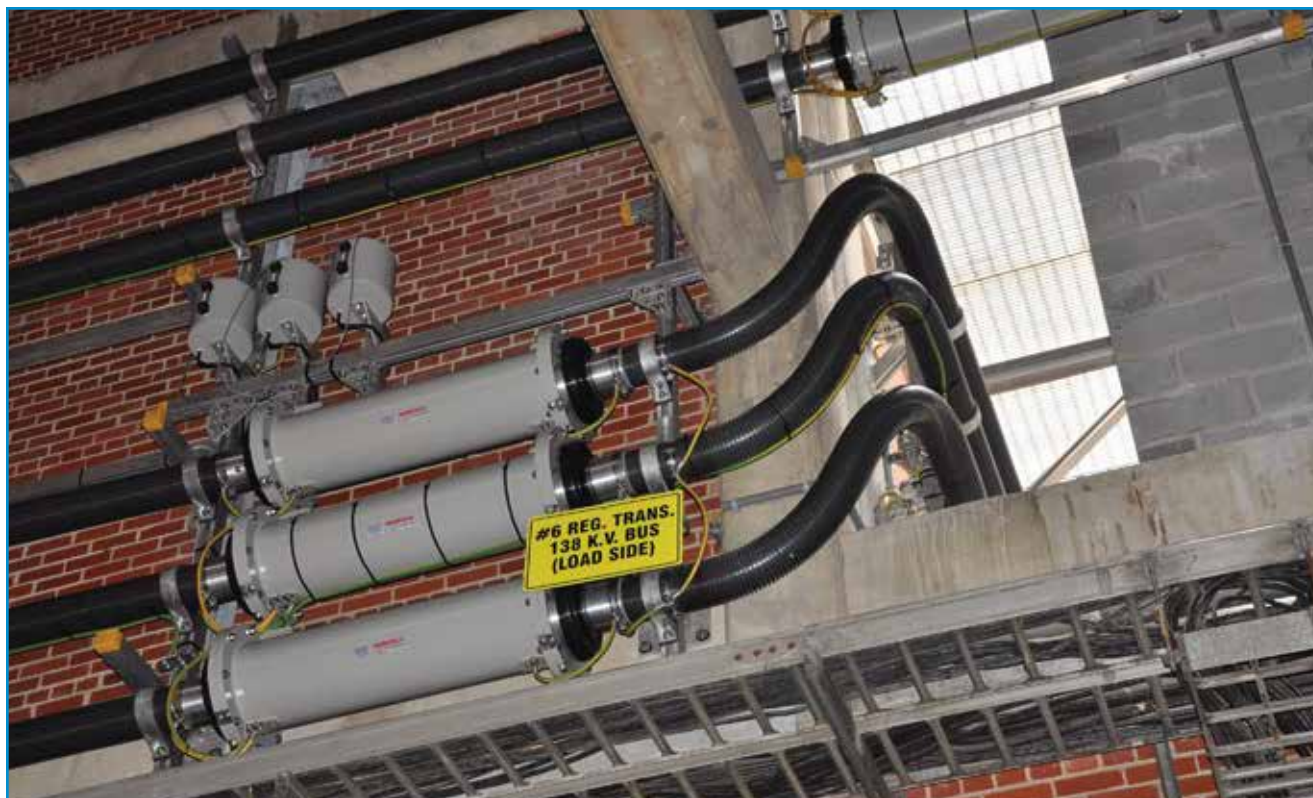
USA - PEPCO Washington DC: 145kV - 1600A
