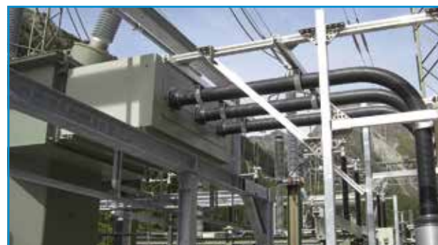
Switzerland - KW Löbbia: 17,5kV - 4000A
